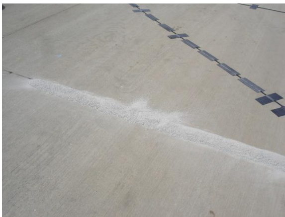
FIGURE F-9 Aggregate ridge after vehicle crossing
